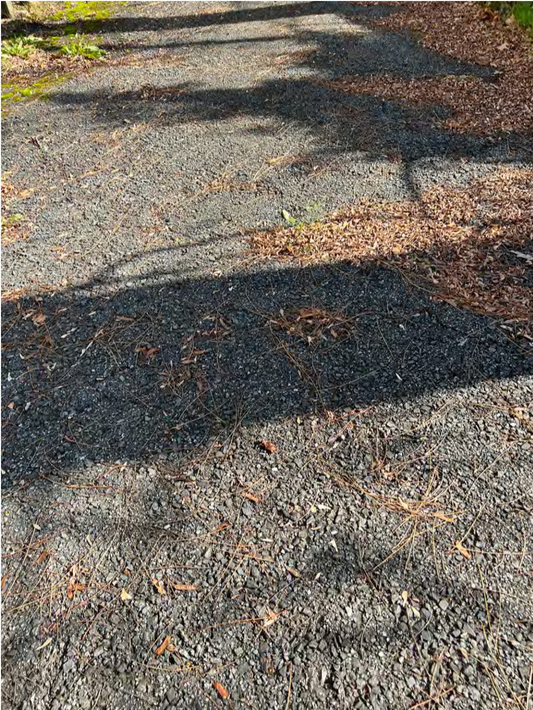
Photo of driveway beginning to decay showing loose aggregate material
