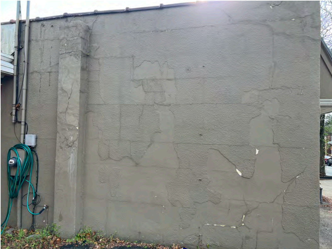
Photo of north building façade indicating peeling paint and cracking.
