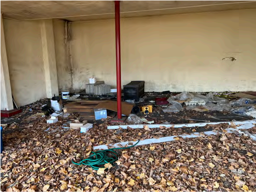
Photo of debris observed at rear of building. Possible presence of mold also indicated on building walls.
