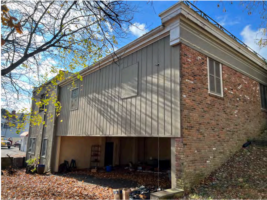
Site photo of rear of building and northerly façade with evidence of debris below the main floor.
