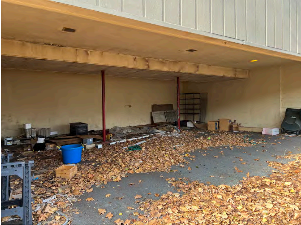
Photo of debris observed at rear of building. Possible presence of mold also indicated on building walls.
